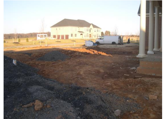
Soil compaction from construction activity.
